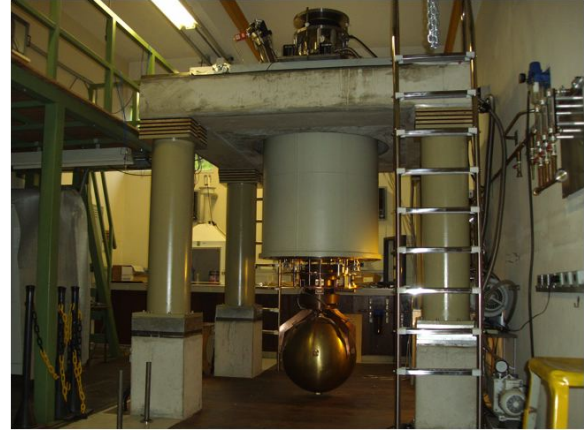
Fig. 6. The sphere was raised about 1.5 meters and immobilized. Beneath it a wooden floor was mounted, which made the assembly work easier. Two nine steps swimming pool ladders were built to provide access to the top of the detector.
